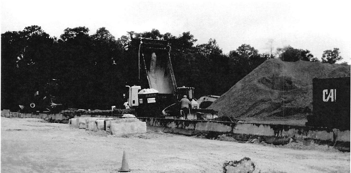
Example of washing down of batch trucks and sand hill: 750 Eastport Road
